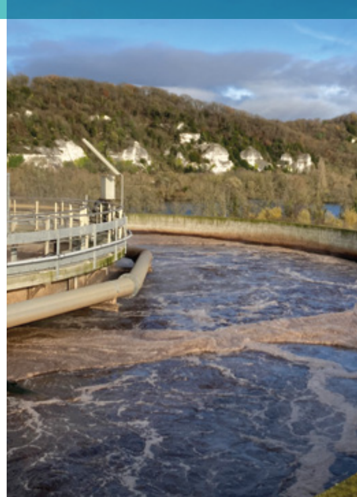
Biological wastewater treatment in the activation basin
