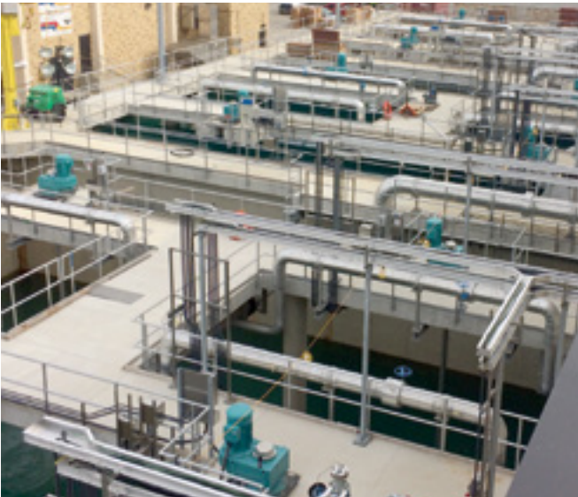
WWTP DC Water Blue Plains, USA
