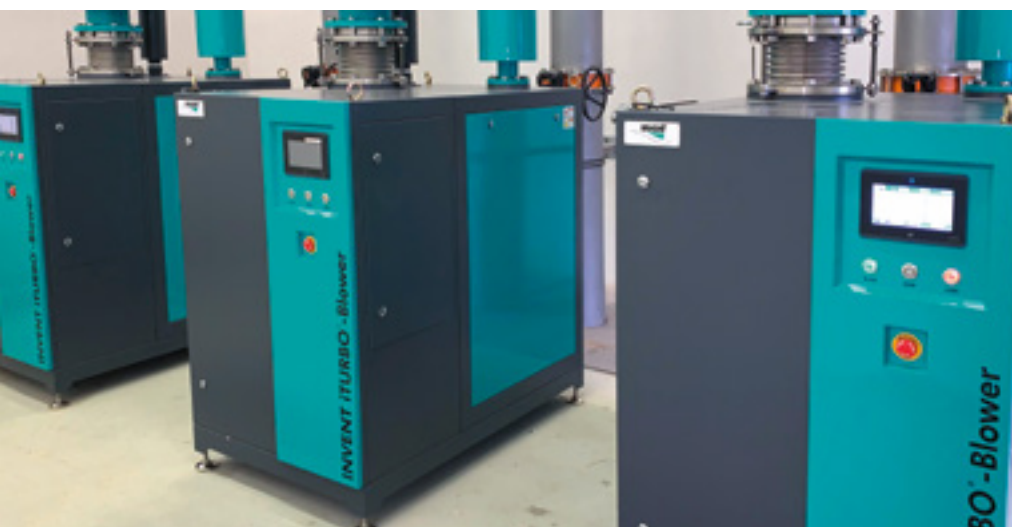
iTURBO®-Blowers in a municipal wastewater treatment plant in the Czech Republic
