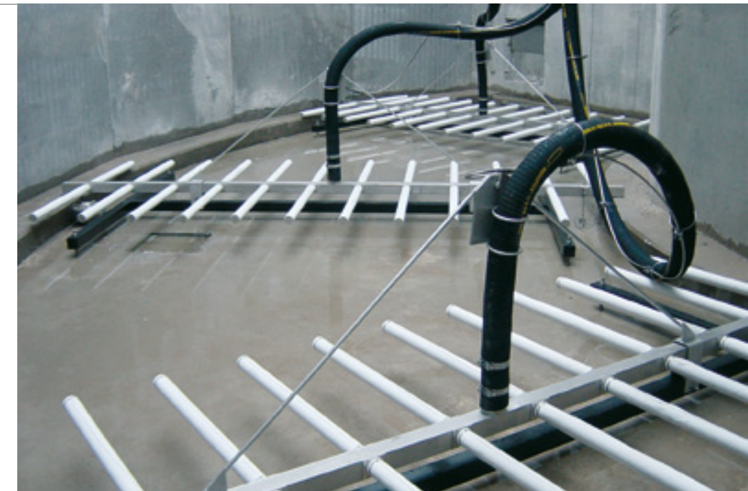
Lift-out version of the TEX-FLEX® -Aeration System on an industrial wastewater treatment plant (pulp and paper industry)
