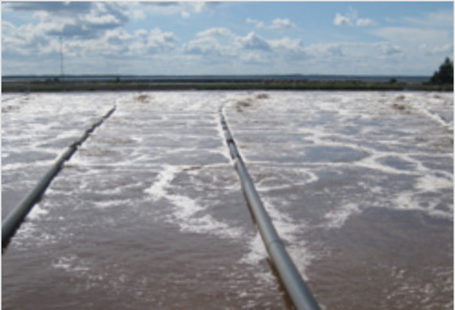
WWTP Stora Enso, Skoghall, Sweden
