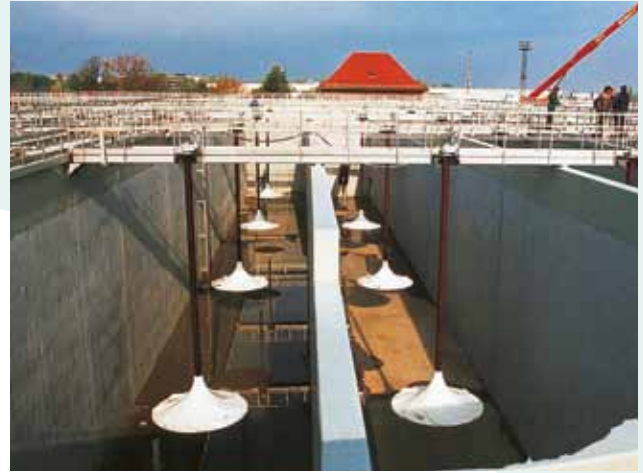
7 out of 33 HYPERCLASSIC® -Mixers in the wwtp Berlin-Stahnsdorf, Germany
